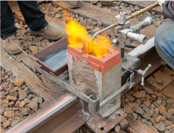
Internal rail flaws are repaired without removing an entire section of rail with thermite head repair welding technology. This lowers the risk of rail defects in the track repair process.
