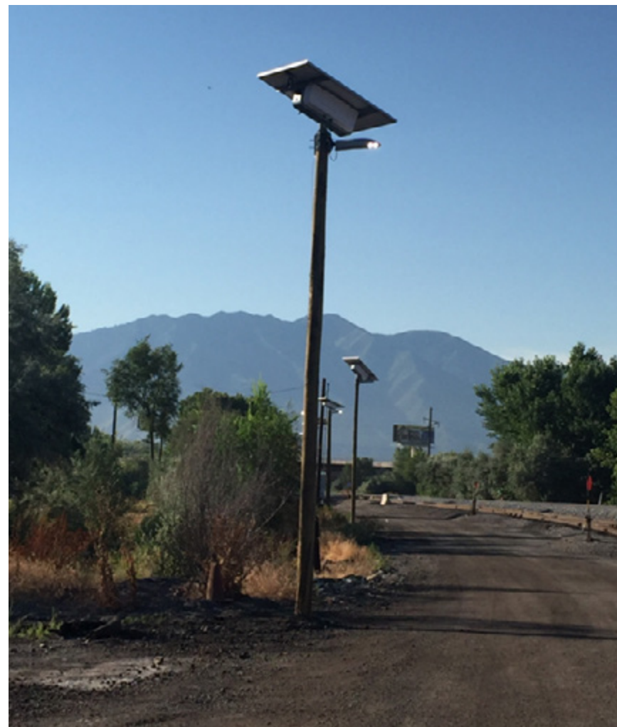
New solar LED lights help train crews safely build trains at night in Utah's Provo Yard.
