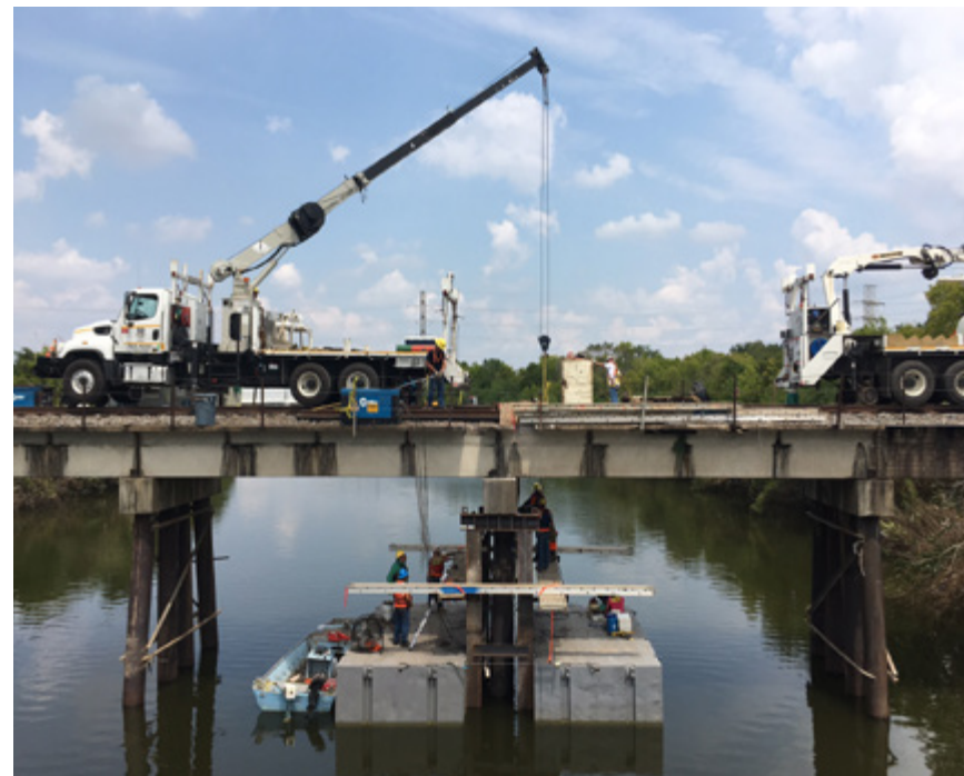
Bridge employees use a truck crane to repair a pier in Houston, Texas.
