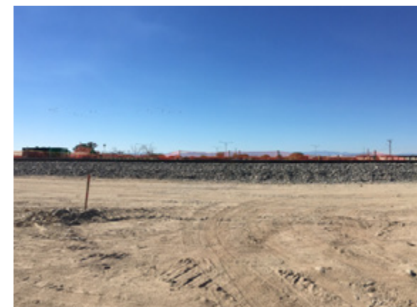
A shoefly was constructed to route train traffic away from the geyser.
