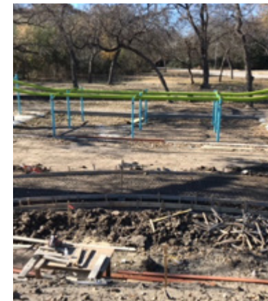
Dream Park construction began in September with equipment installation, followed by rubber surfacing, sidewalk and fence work.
