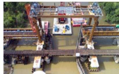
The movable lift span over the San Bernard River Bridge was slid into place in one outage, preventing nearly a dozen additional outages.
